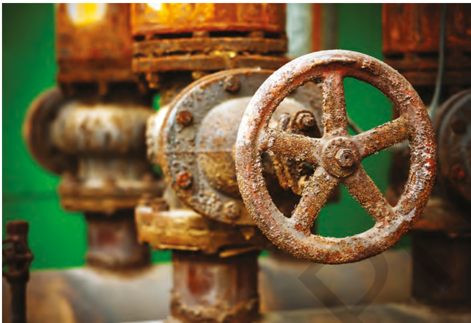
FIGURE 9.5.1 Corrosion is causing water to leak in these pipes in a pumping system.
