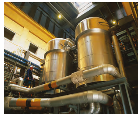
FIGURE 9.4.16 Interior of the PRODE fuel cell power station in Milan, Italy, which began operating in 1992. The cells use hydrogen as the fuel and phosphoric acid as the electrolyte. The fuel cells can produce up to 1.3 MW of electricity.
